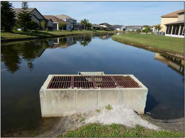
Stormwater Drainage Control Structure
