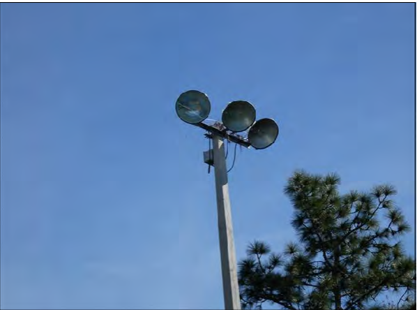
Tennis Courts Lighting
