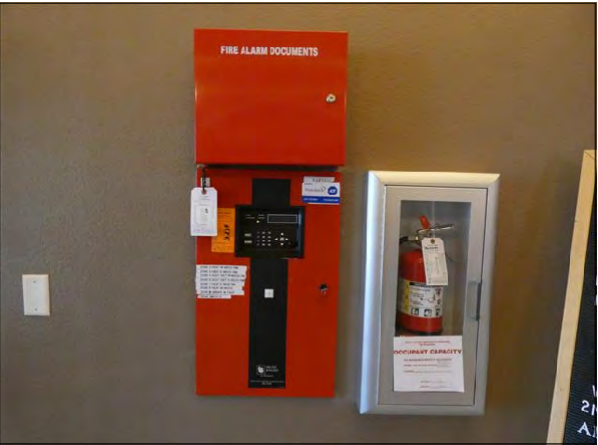
Clubhouse Fire Alarm
