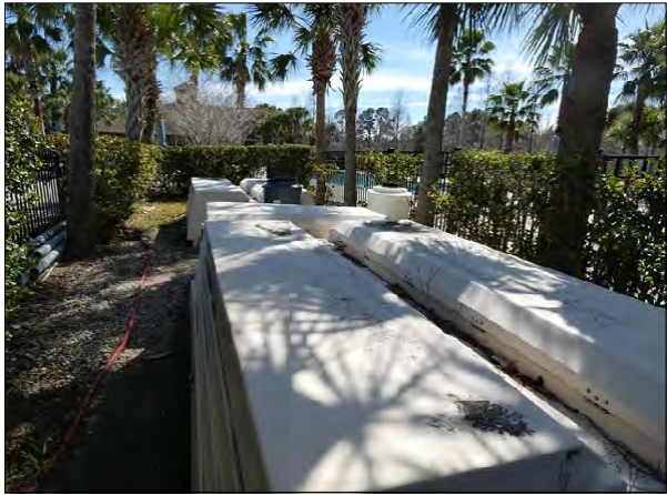
Pool Equipment Housing Boxes
