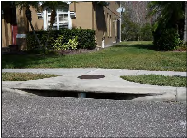
Stormwater Drainage Curb Inlet
